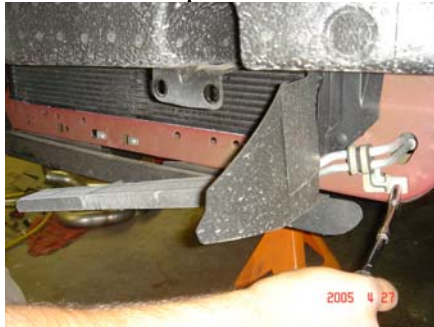
80. Relocate power steering cooler line clip to other slot in radiator support.
